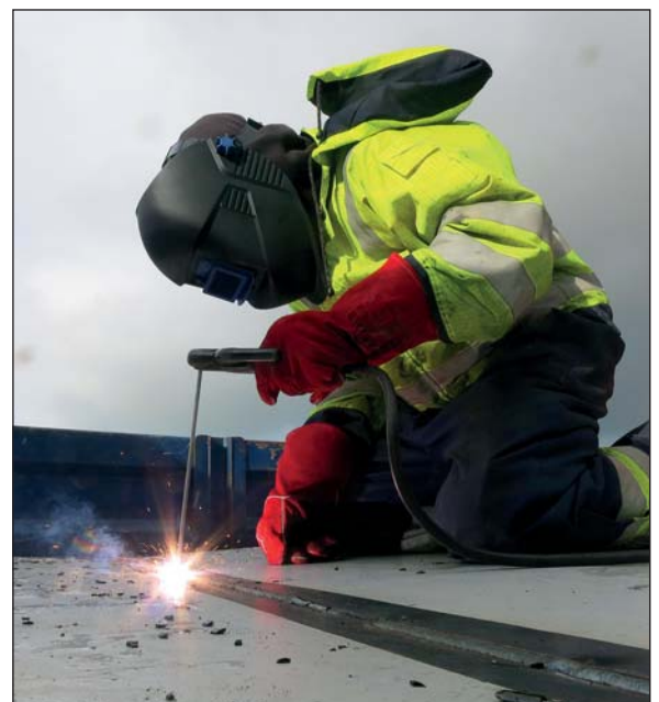
Hydrex certified dry welder preparing one of the larger blanks for installation.
