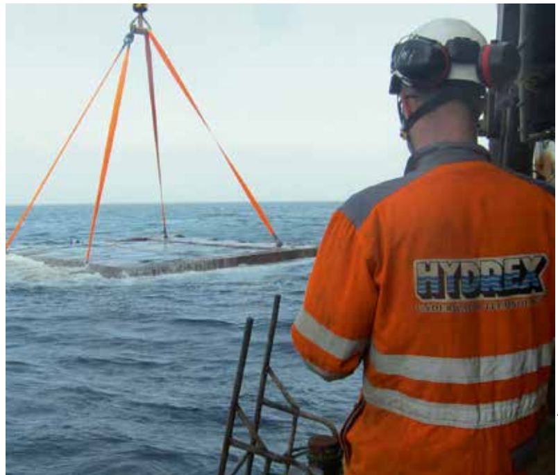
Hull repair on a drill ship in the Gulf of Mexico in 2018
