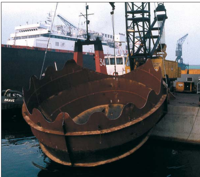
Hydrex took on the job of designing and constructing a shell to cover the damaged bulbous bow.
