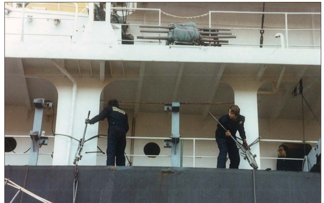
Wire pullers were used to keep the cofferdam in place during the
