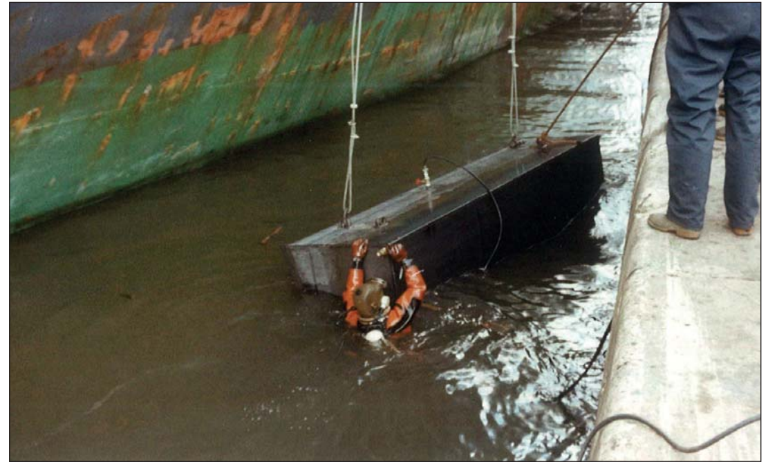
The cofferdam filled with water, allowing it to sink. Later it was dewatered with compressed air and gained positive buoyancy.
