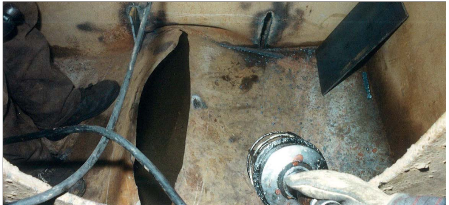
The damage in the double bottom of the engine room was severe.
