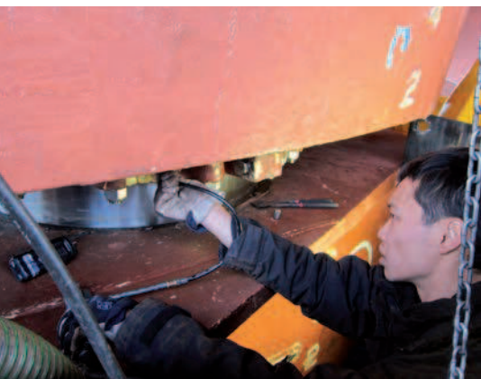
Hydrex's new Mobdock takes the drydock out of the rudder repair equation
