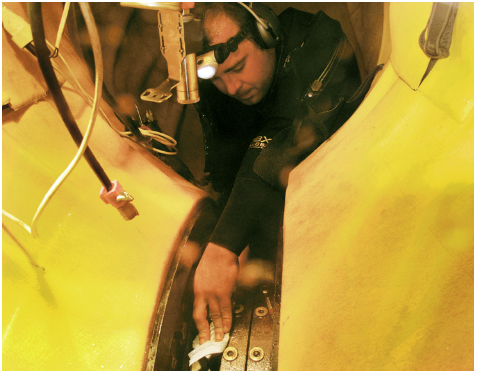
Hydrex can carry out in-situ repairs to seals and bearings (credit: Hydrex)
