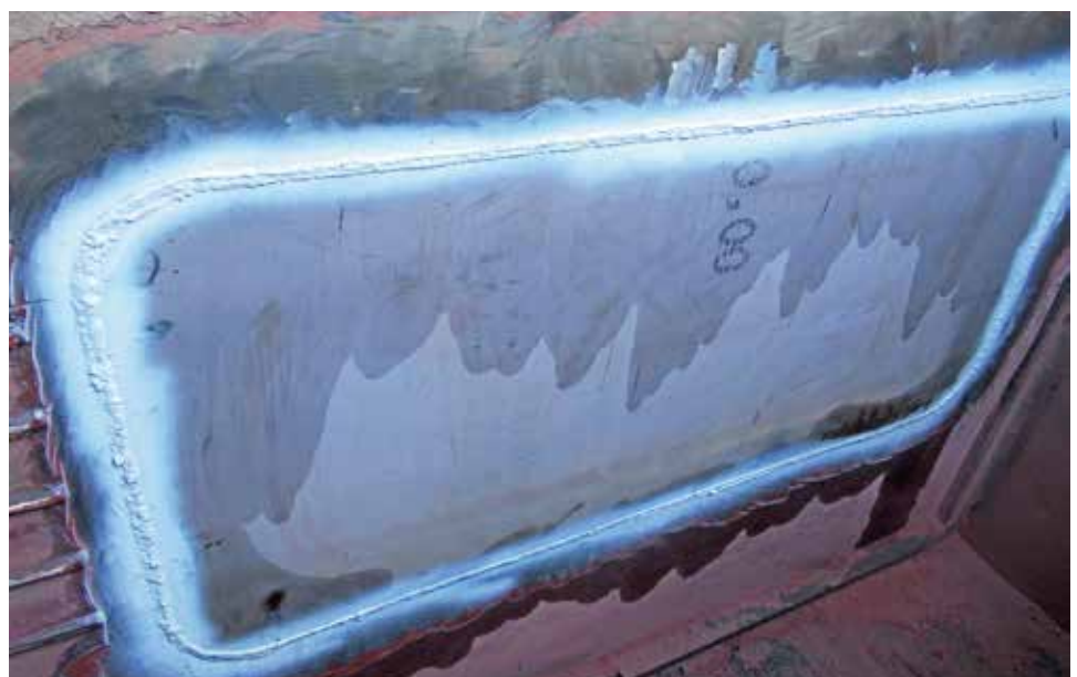
Hydrex secured the insert with a certified weld both from inside the vessel and inside the cofferdam.
