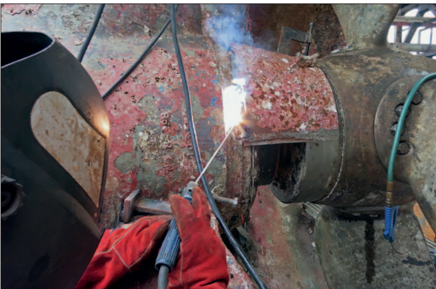
Hydrex certified welder reinstalling the rope guard of portside azimuth thruster in Mexico.
