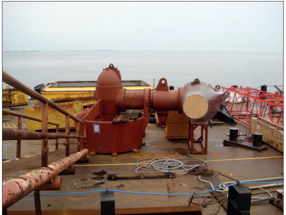
40-ton swing-up azimuth thruster of an offshore crane barge. Behind it the 9x6x2 meter yellow mobdock we designed and constructed for the removal of the unit.
