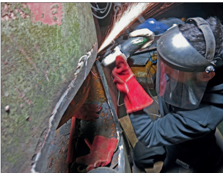
Beveling the edge of the rudder plate to fit the new cover plate.
