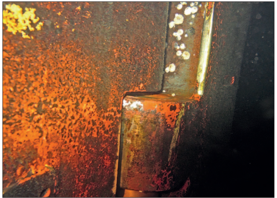
The top hinge of the rudder flap had come loose.
