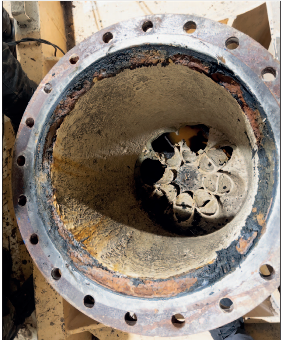
Corroded scrubber pipes can cause severe leaks.
