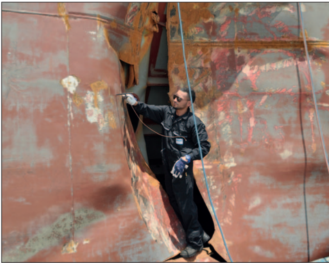
A full inspection of the damage on the bulker in Abidjan
