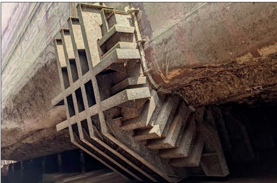
When the ship arrived in drydock, the sheer size of the cofferdam could be appreciated.
