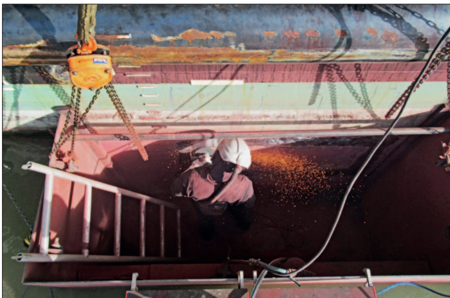
Hydrex welder cutting away the old plating from inside the open-top cofferdam on the ferry Texelstroom.
