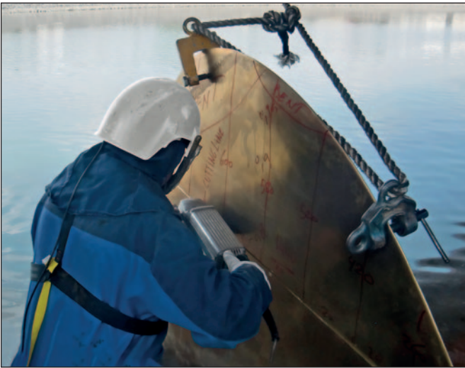
Cutting the opposite blade of the damaged blade to keep the balance.
