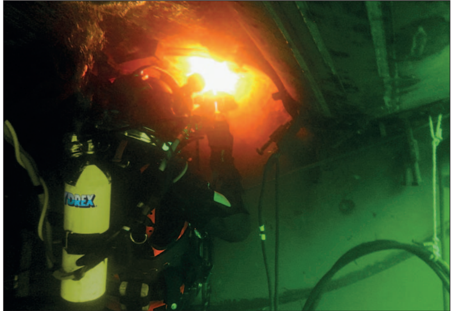
Our teams routinely perform underwater welding work to the highest quality standard.
