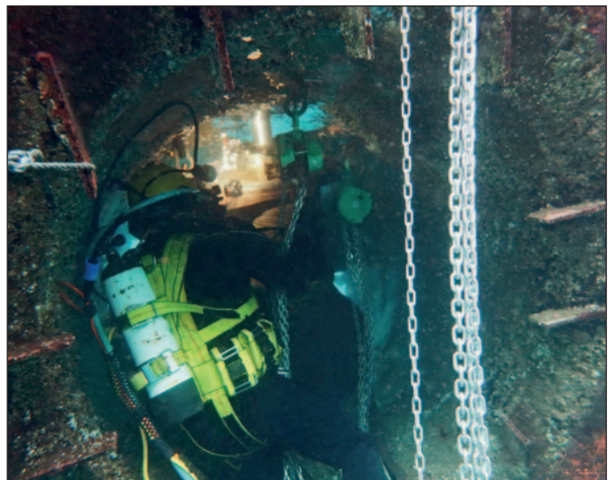
The unit being lined up with the connection to the bow thruster room by Hydrex diver.
