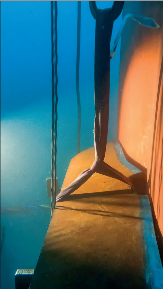
The stiffeners were fabricated using the exact measurements taken during a comprehensive inspection done by our divers.
