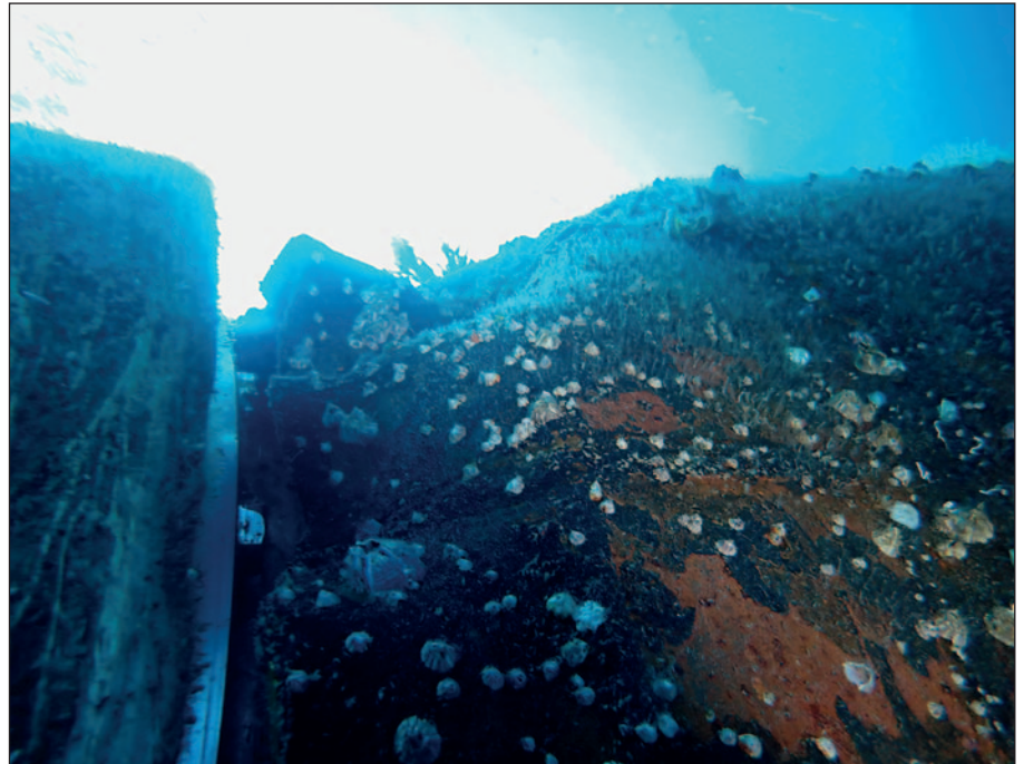
Damaged rope guard prior to being removed and replaced.
