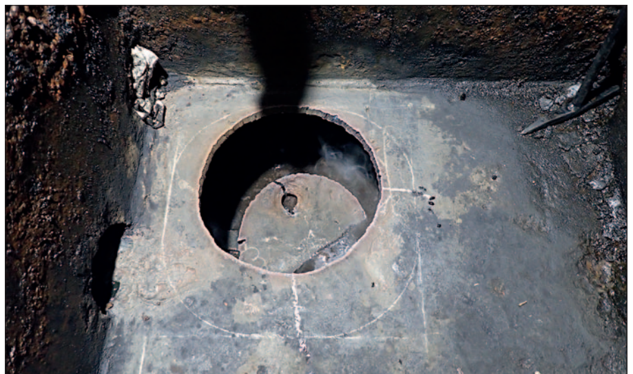
The area where the insert was to be installed was cut away.
