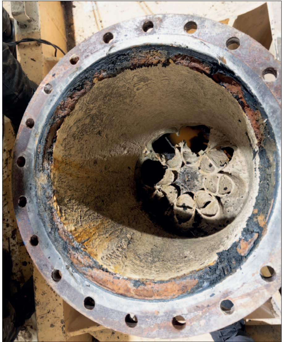
Corroded scrubber pipes can cause severe leaks.
