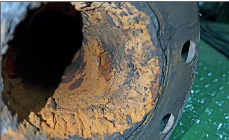
Severely corroded discharge pipe on crude oil tanker in Rotterdam.
